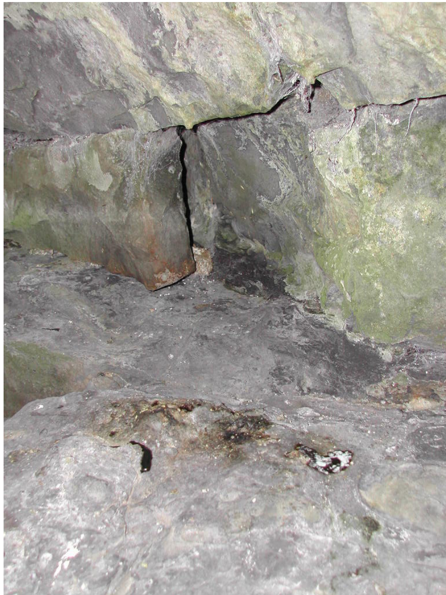
Plate 40 Otter holt comprising of a hole in the stonework of a road bridge.
